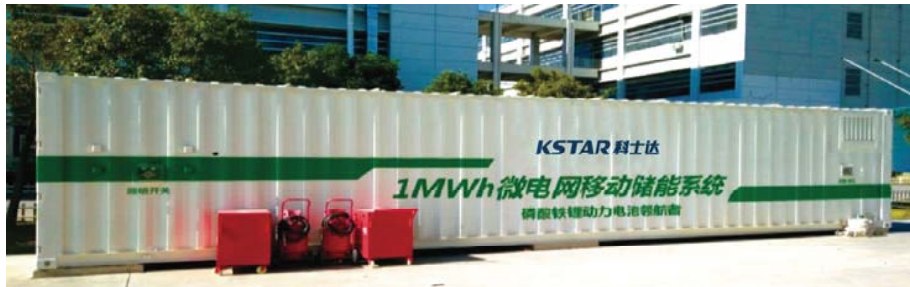
► 3MW/12MWh BESS Demonstration Project in Shenzhen
