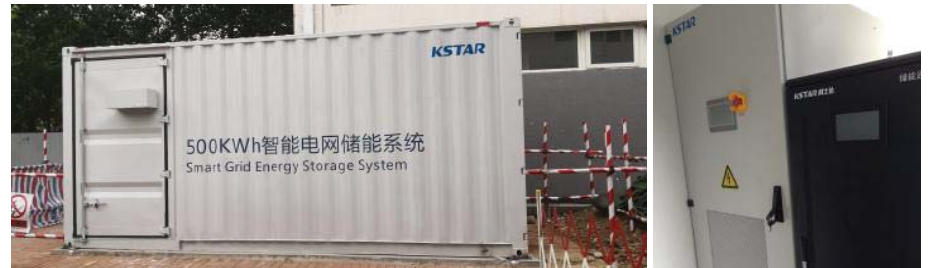
► 500kWh Multi-energy Complementary Project of Beike Industrial Park
