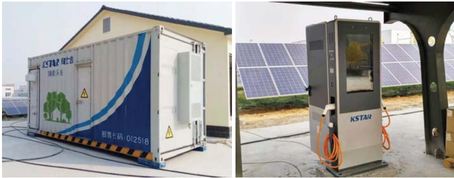
► 50kW/200kWh BESS for EV Charger Station in Hebei
