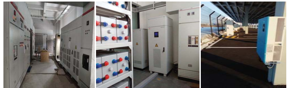
► BESS for EV Charger Station in Harbin
