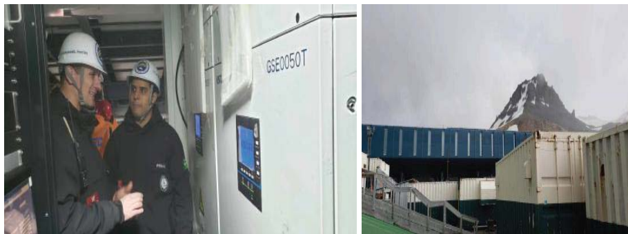
► 300kWh Storage Project of Brazilian Military Antarctic Research Station
